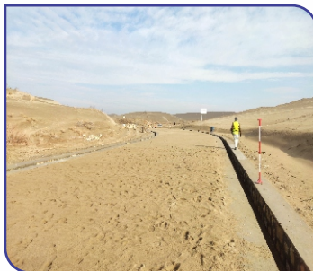
Figure 1: Existing Subgrade of Loose fine sand on the Shortepa District Road.
