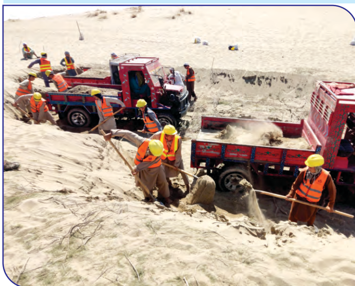
Figure 1: Excavation and disposal works using labour at the Road rehabilitation of Shortepa road
