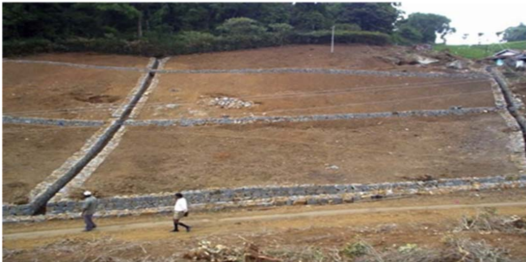
Picture 1: Water drains with water revetments (Source: DoA, Collection of Presentations)
