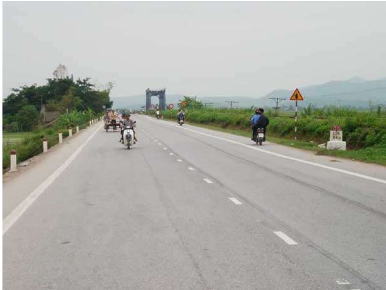
Km 294 on NH 1 close to Ninh Binh. This section has been identified as part of the first year maintenance programme. Works will mainly consist of resealing the surface.
