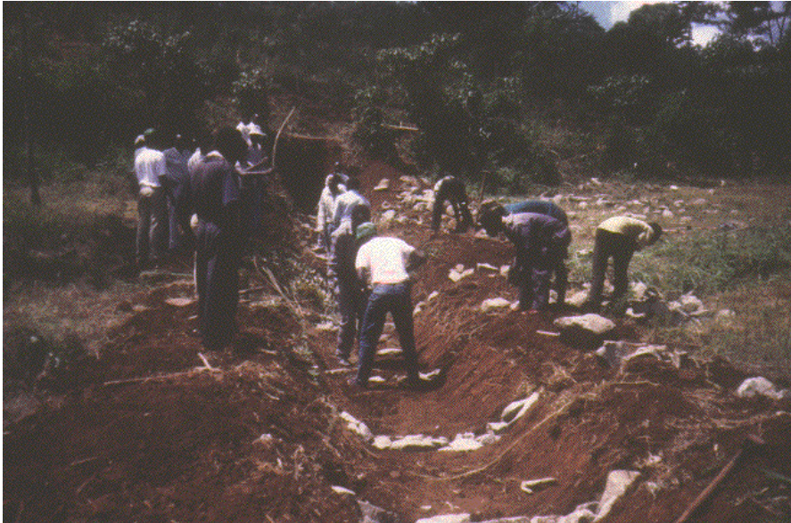
Construction of artificial waterway to convey water safely to a disposal point
