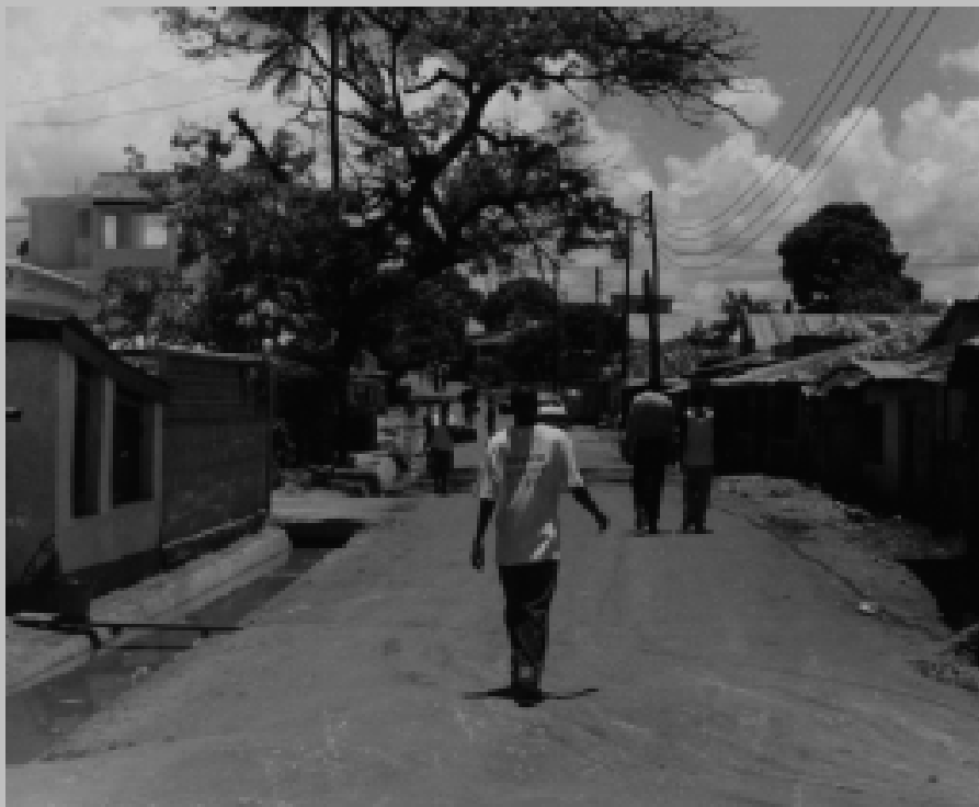
Storm water drain and access road in an unplanned settlement constructed through community contracts, Hanna Nassif.
