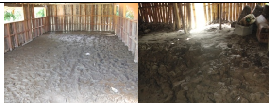
Roroni community kindergarten school and community hall filled with mud and needs clearing.
