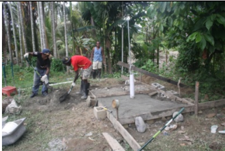
Workers involved in rebuilding of the destroyed community wash room and well in Papangu. The community purchased the cement and plumbing materials with their own funds.
