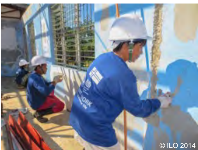
Workers patch up a classroom's wall prior to its roof being installed.
