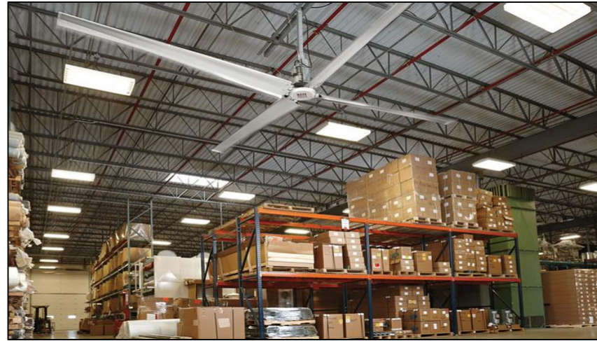
Energy efficient HVLS fans
