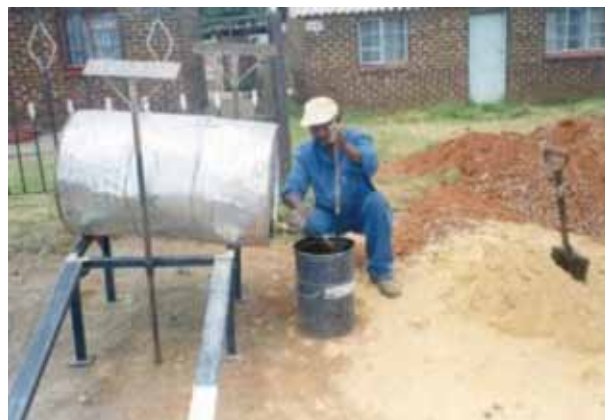
Steel frame stand for decanting emulsion
