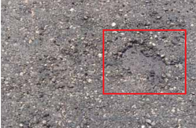
Mark the area of the pothole
