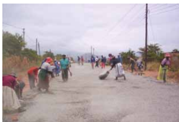
Un-even spreading of aggregate
