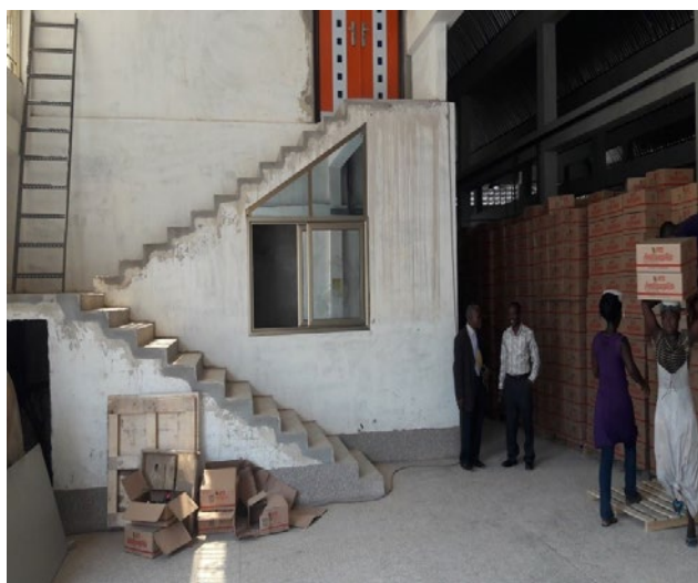
Before: no railings on the staircase meant a safety hazard
