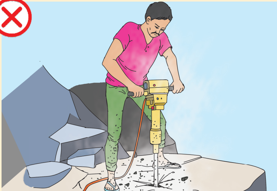
Unsafe ways of handling jackhammer
