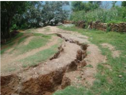
Gully in road surface
