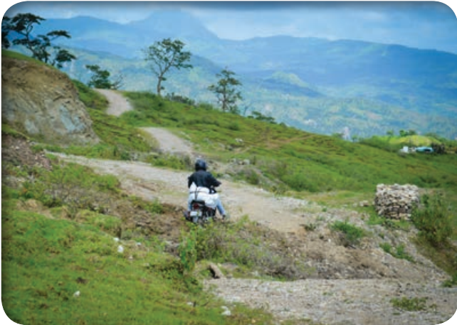
Rural roads are in poor condition
