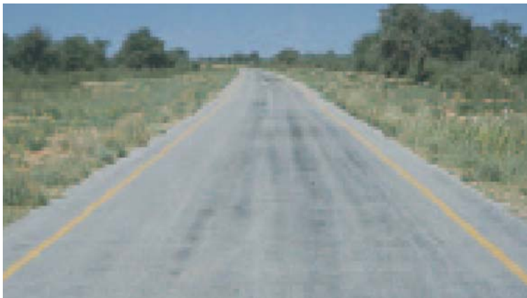
Gambar 22: Otta seal road after 9 years of operation and without maintenance
