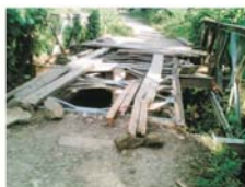
Muddy road and rudimentary bridge in Nias suffering from lack of maintenance
