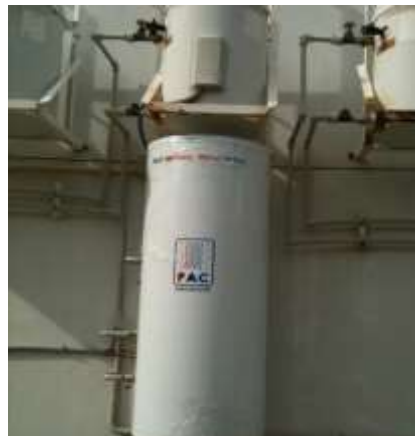
New heat recovery water heater
