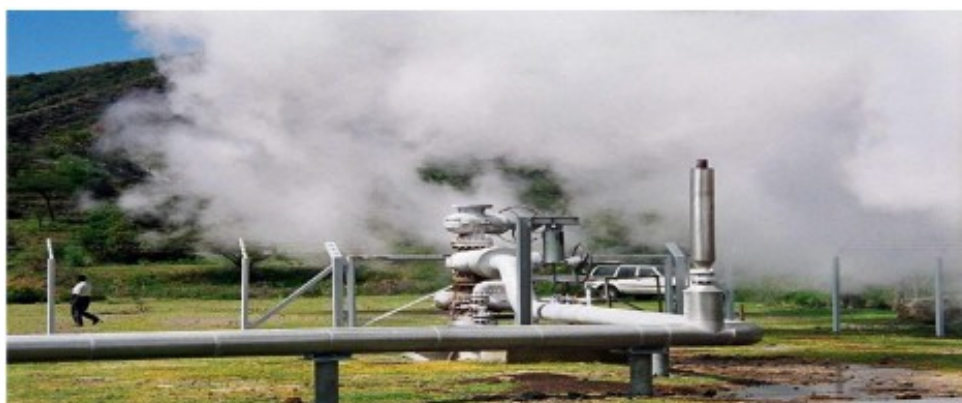
► Fig 5. Aluto langano geothermal plant
