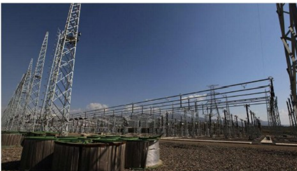
► Figure 7. High voltage(500 KV) transmission line in Ethiopia.
