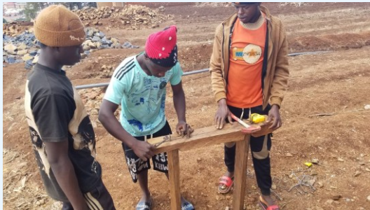
Workers doing iron bending in a building site in Bamenda working without any PPE
