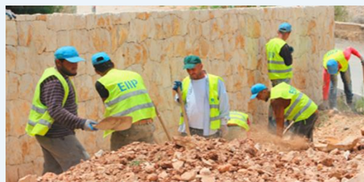
Photo 7: Building storm water drains in Mount Lebanon Area
