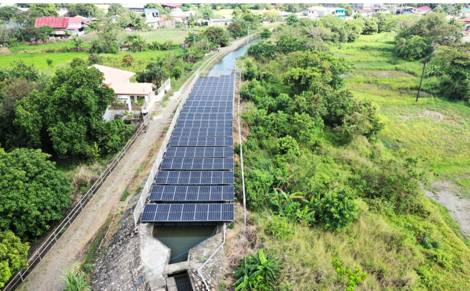
Kapatiran Solar Pump Irrigation System at AMRIS North Main Canal in Sampaloc, San Rafael, Bulacan. Photo: © NIA Central Office
