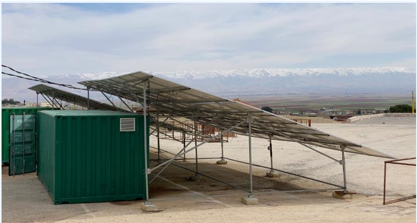
Portable solution installed in the Union of Cooperatives of Deir El-Ahmar
