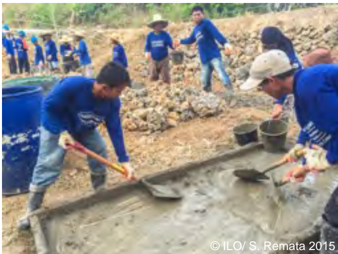
Workers prepare the cement that would hold together the stones that would form the causeway's riprap.
