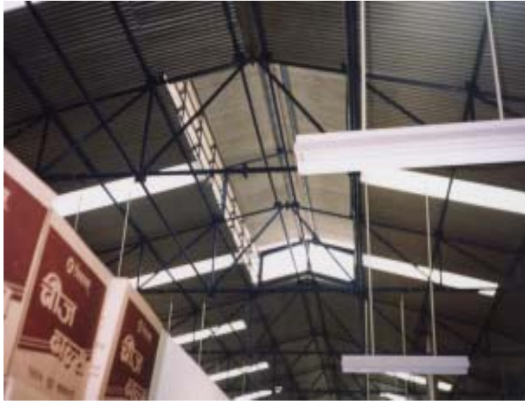
Skylights for utilizing daylight.
