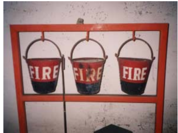
Providing fire buckets near a workshop.
