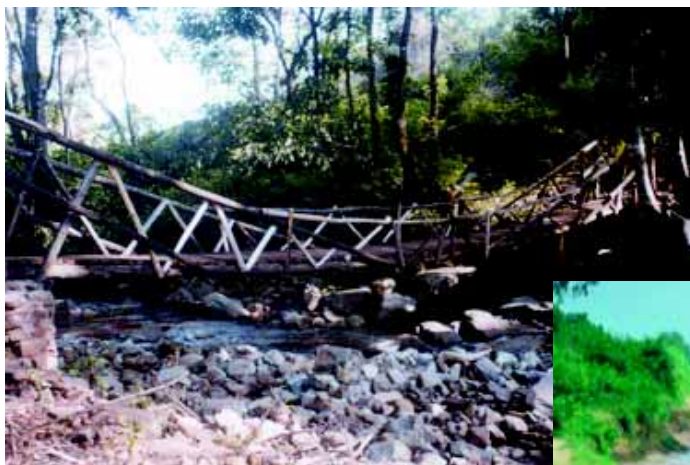
Poor access – increases level of hardship on the community
