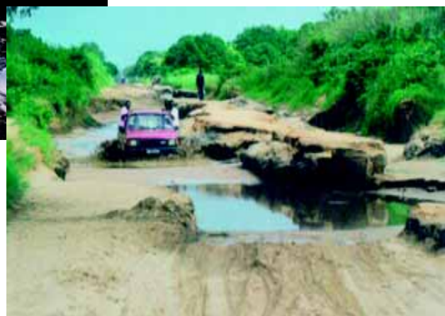
Poor access – a barrier for sustainable development
