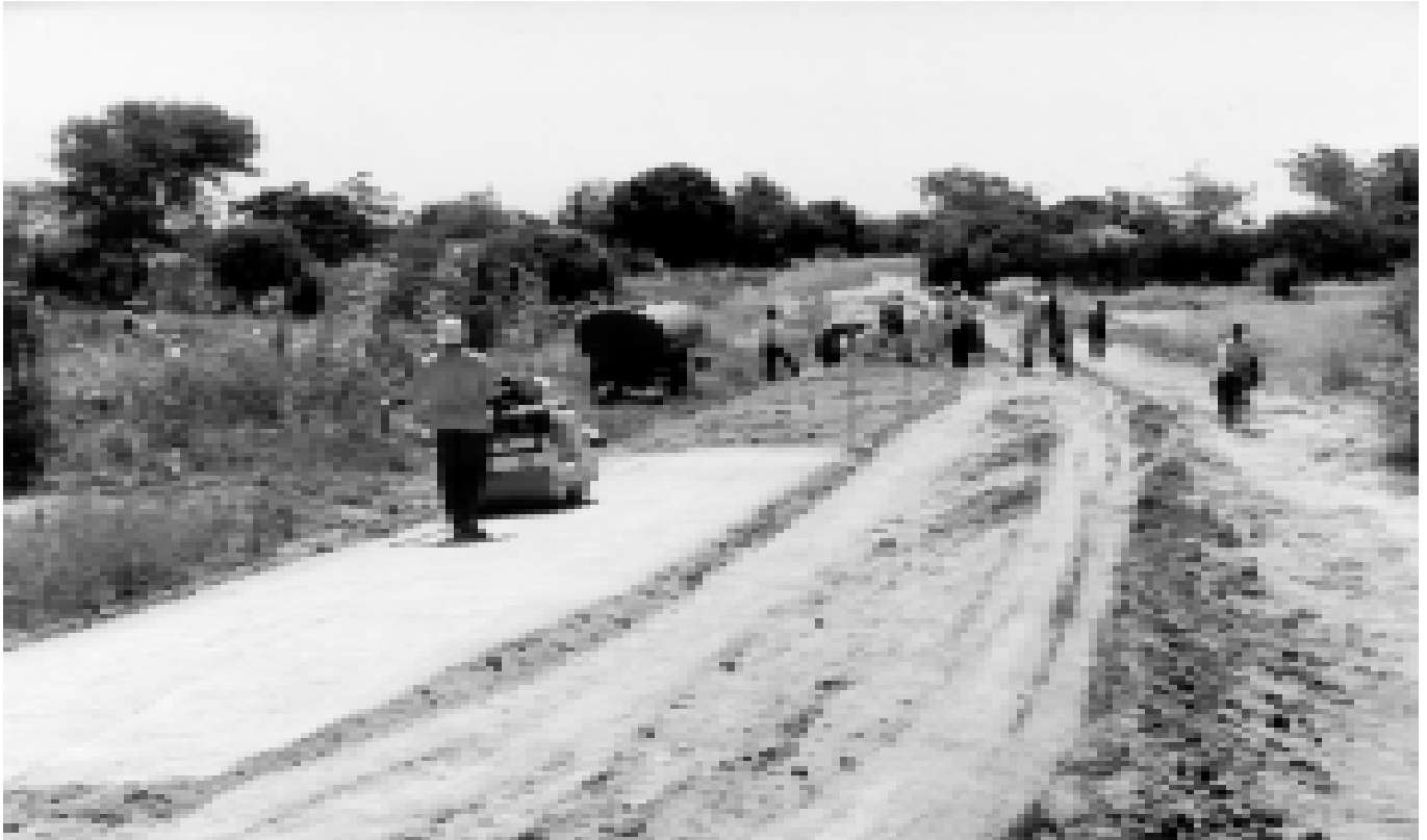
Rehabilitation work in progress on the Lugeye-Kigangama road in Magu district, Tanzania
